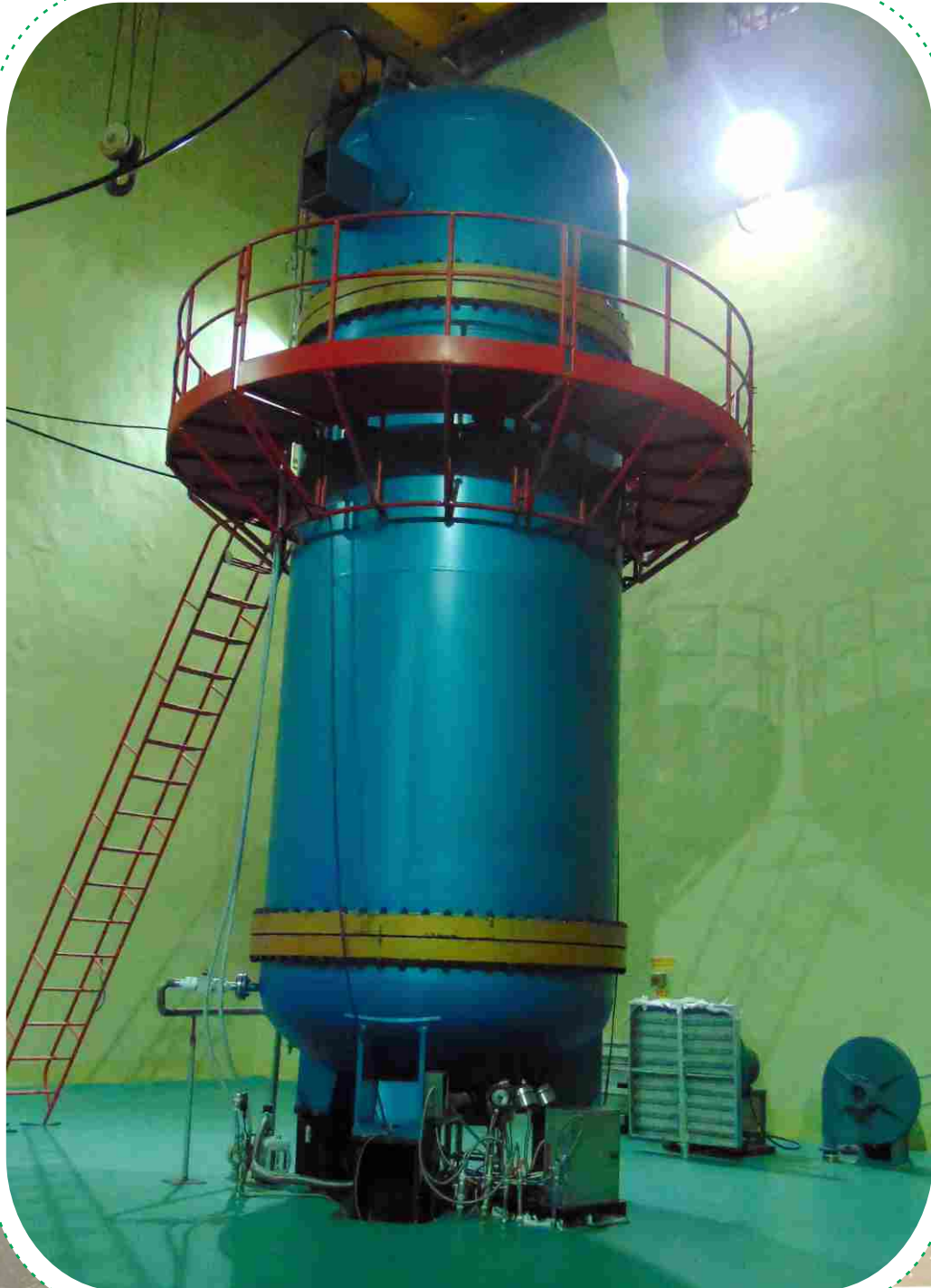
Electron Beam machine at Khatalwada plant.
